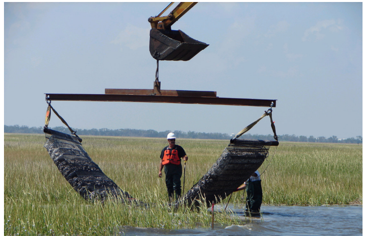
Installation of Gabion Mats (one of the three techniques being used on this project) along the north shore of Lake Barre.
