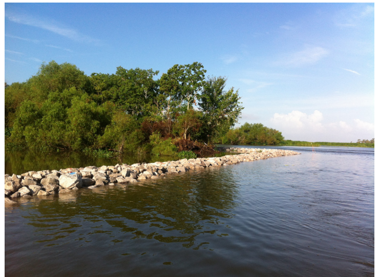
Typical section of forshore rock dike construction as viewed from the GIWW near Copesaw Canal. The typical rock construction includes a lightweight aggregate core to prevent the structure from sinking in these soils that are very organic and have very low load-bearing.
