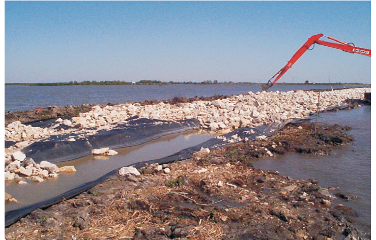
The narrow, eroding shoreline of Bayou DeCade was reinforced with rock in order to help restore the hydrology of the Brady Canal area.
