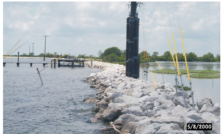
Much time and effort were spent coordinating with petrochemical and electrical power suppliers to ensure that existing systems were not damaged and that customer supply was not interrupted as various project features were installed.
