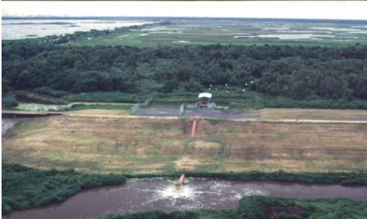
A Bayou Sauvage pump station in operation, facing west. It is removing water from the project area, depicted in the upper portion of the image.
