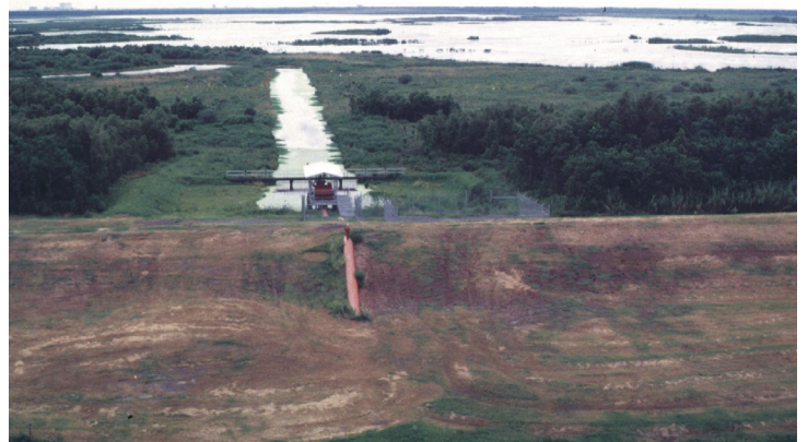
A Bayou Sauvage pump station, facing west into the management area.
