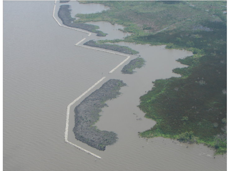
Segmented rock breakwaters such as the one constructed above will provide protection for White Lake's eroding shoreline.
