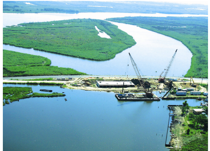
The construction of the Black Bayou Culverts will help the flow of floodwater out of the Calcasieu-Sabine basin while preventing saltwater intrusion from Calcasieu Lake.
