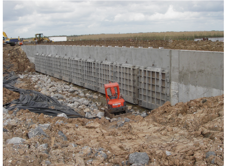
The construction of Black Bayou Culverts included ten 10 foot by 10 foot concrete box culverts under Highway 384 to help with drainage from Black Bayou to the Calcasieu River. The construction of Highway 384 had altered and effectively blocked the original drainage system.
