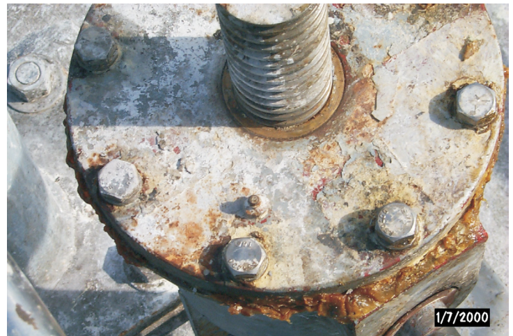
The salty environment of the project area leads to severe corrosion of unprotected pipes, fittings, and valves. This corrosion can eventually leave the water control structures inoperable.
