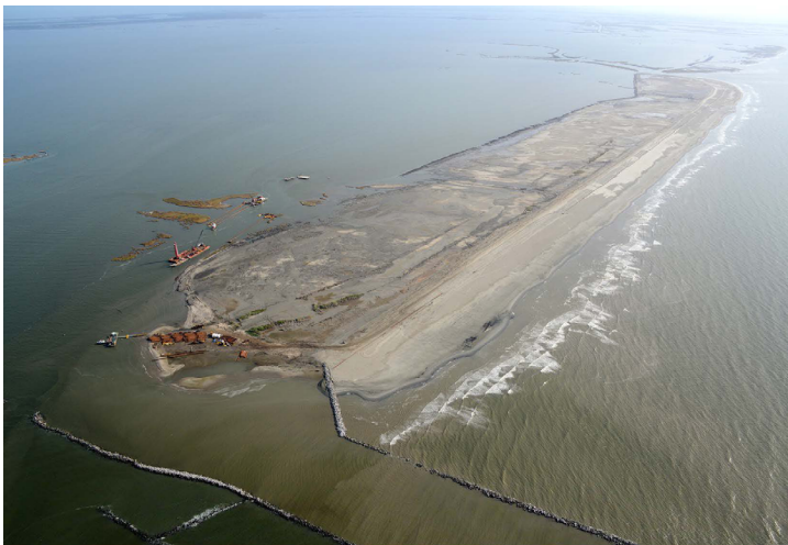
Pelican Island after completion of major construction activities. Large equipment in the lower left of the photo provide a sense of the scale of the project.
