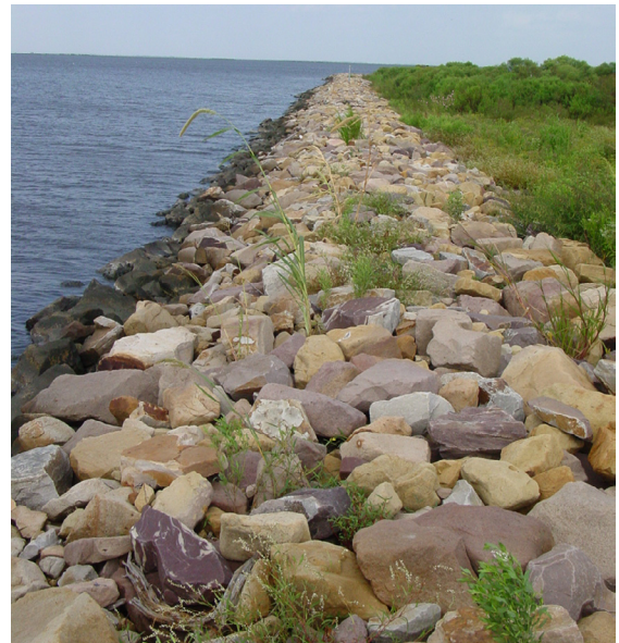
Five years after construction, the constructed rock revetment has proven to be very effective at eliminating shoreline erosion.
