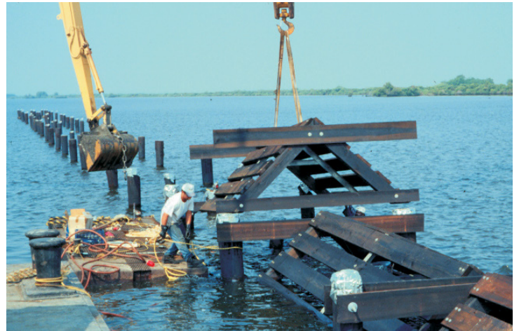
Installation of an erosion control structure during Phase 1 of the Lake Salvador restoration project.
