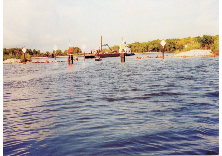
Weirs constructed with a boat bay aid in the effective management of hydrology while still allowing the passage of small boats and vessels.
