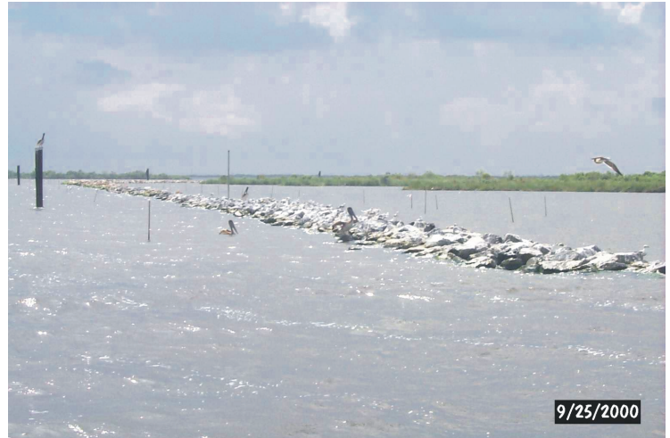
The constructed rock breakwater located in Bay L'Ours will assist in reducing wave energies before they impact the shore and will also arouse the curiosity of local waterfowl such as these pelicans.
