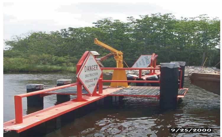
This winch which is permanently attached to the variable crest, water control structure located right off Briton Canal, will help to configure the structure according to a pre-determined water management plan.
