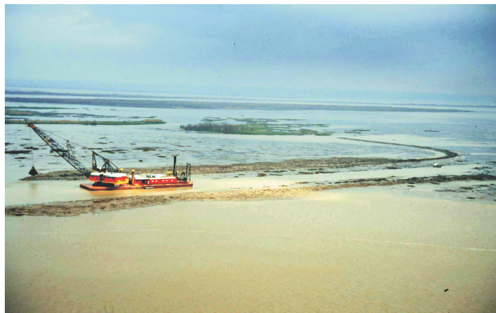
A bucket dredge is shown removing sediment from a shoaled-in channel in order to help reestablish water and sediment flow within the Atchafalaya Delta.
