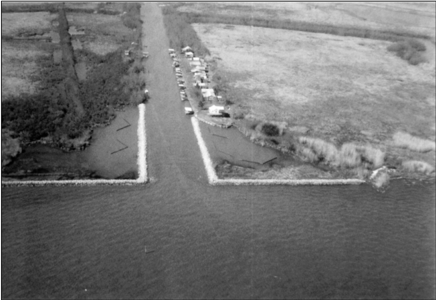
Figure 2. Boston Canal/Vermilion Bay Shoreline Protection (T/V-09) rock breakwaters and sediment fences at the mouth of Boston Canal.
