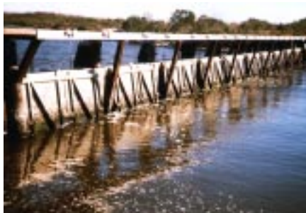
Flap-gated water control structure at Montegut (TE-01).
