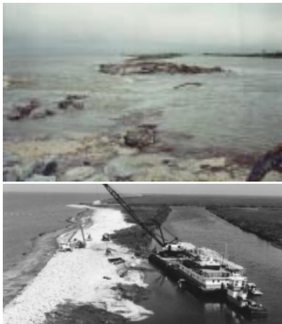
Closing a breach in the shoreline at the Point Au Fer Canal Plugs (TE-22) project.
