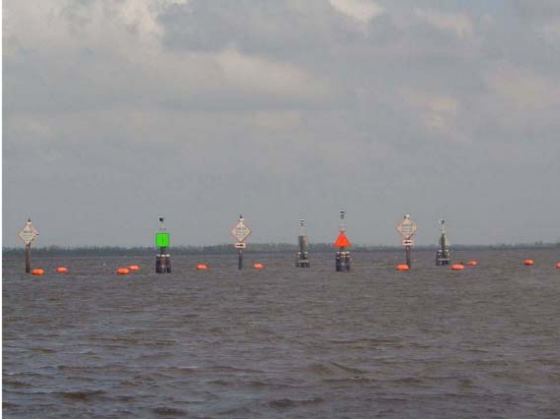
Photo #2 – Goose Bayou Canal Weir. Approaching the Goose Bayou weir from the Barataria Waterway side, looking across the weir boat bay toward the Pen. Warning signs and navigation aids are shown on either side of channel through the boat bay. Note the damaged lights.
