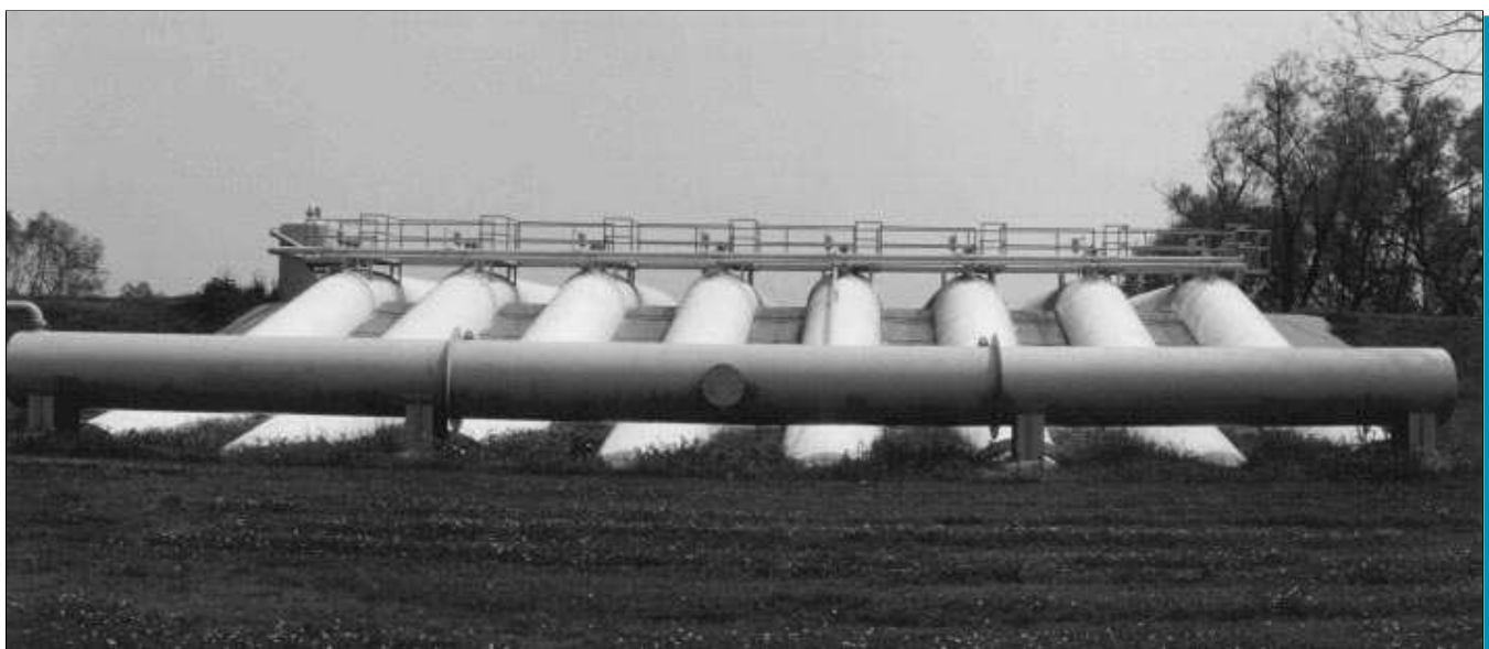
A view of the Naomi Siphon in Plaquemines Parish. Similar technology and structures will be used in the Myrtle Grove Siphon Project – one of two large-scale, freshwater diversion projects endorsed by the CWPPRA Task Force in February.
