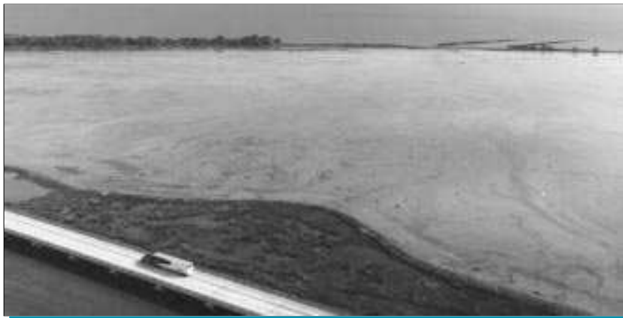
The LaBranche Wetlands shortly after the sediment transfer phase of construction. Since that time, the area has been seeded with Japanese millet. Further plantings will be completed in the project area by 1999.
