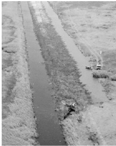
Construction contractors reinforce a canal bank with rock. Similar work will occur at the Sweet Lake-Willow Lake project.
