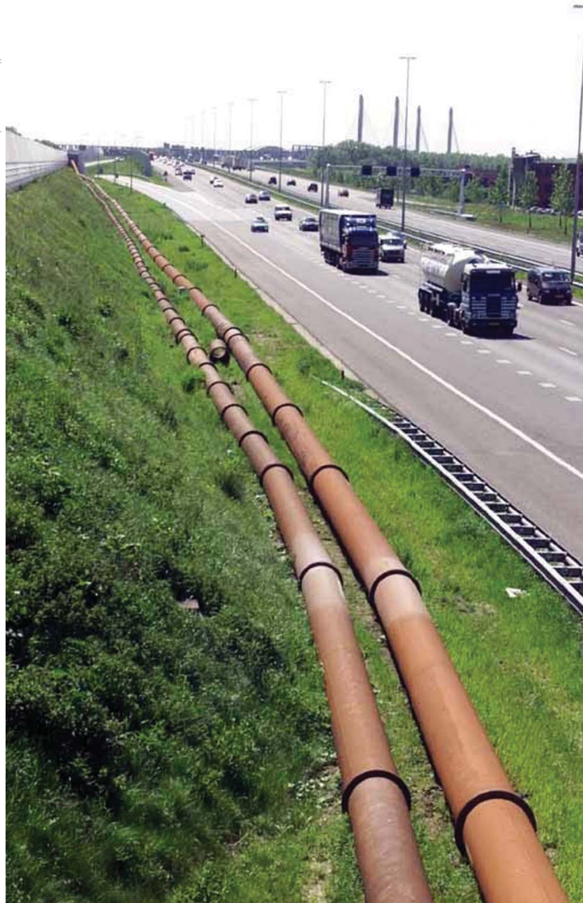
To build one of the largest infrastructure projects in Dutch history, sediment was pumped through 100 miles of pipeline to create the bed for a two-track freight railway.
